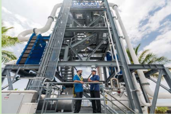
Hawaii's 100kW Class Facility
